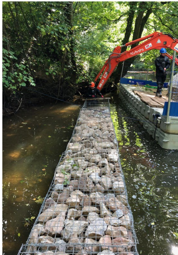
Gabion baskets filled with rocks at Newton St Cyres, TMS
