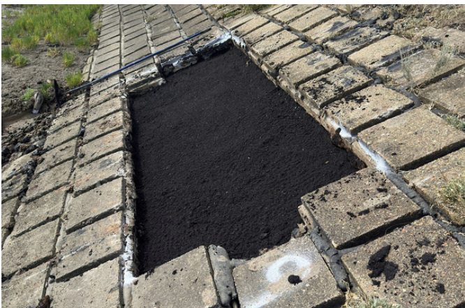
LSA used as void filler where concrete blocks have failed
